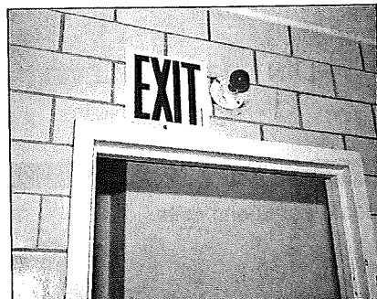
Figure 3.8: Mark each evacuation route with signs and lights.
