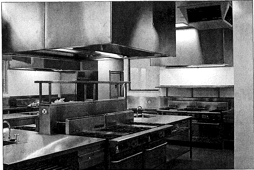
Figure 3.11: A hood ventilation system is installed over cooking equipment to remove vapors, heat, and smoke.
